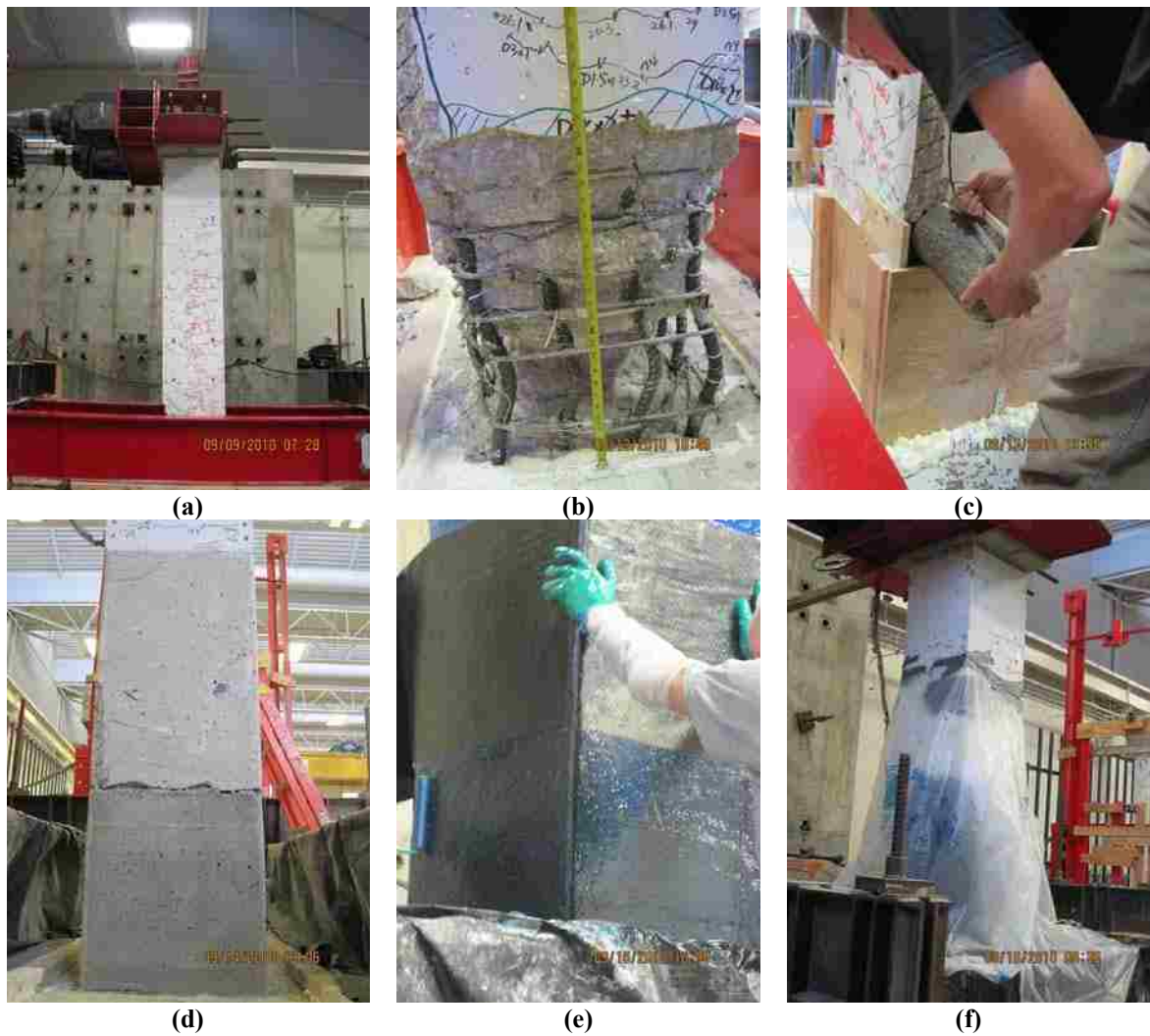
Fig. 11. Repair procedure. (a) Column after straightening, (b) column after loose concrete removal, (c) repair mortar placement, (d) surface preparation, (e) CFRP application, (f) curing process.
